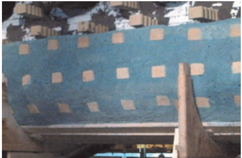
SAVAGE RAM 70-M BLUE rammed in a bull nose of a reheat furnace.
