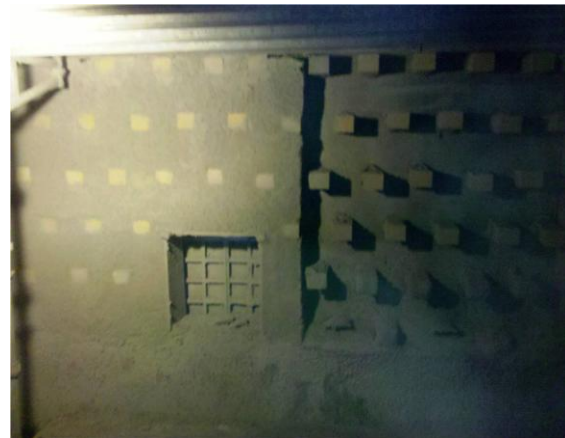
A wall recently shot with Q-TEK 32 GM. Overall appearance was of a wall rammed with plastic. The result was also the same with a strong, phosphate bonded monolithic lining.
